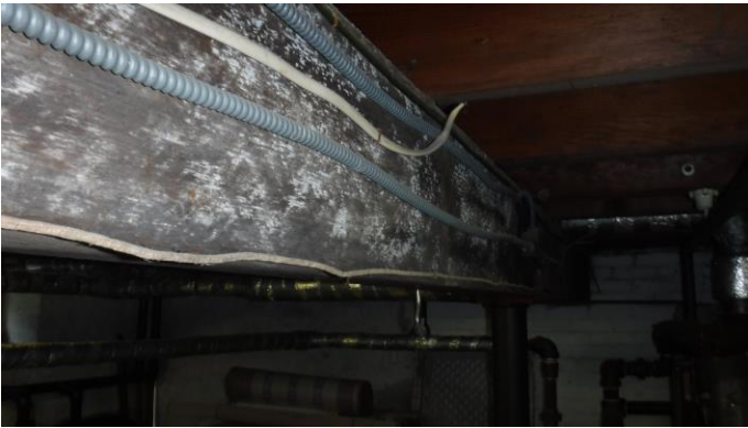
Confirmed mold growth on basement main beam.
