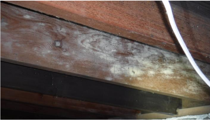
Apparent visible mold on crawl space joists.
