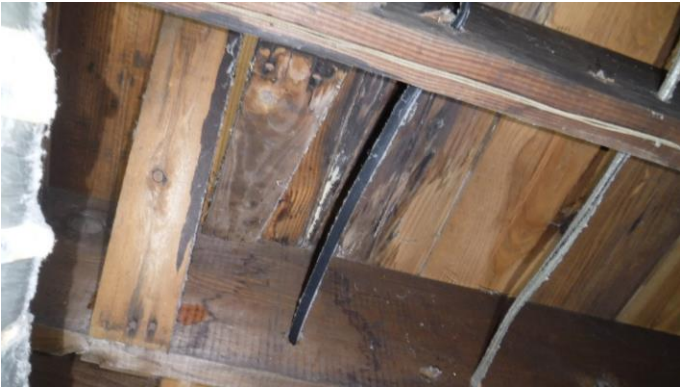
Apparent visible mold on basement subfloor.
