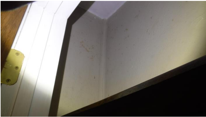
Apparent visible mold on 2 nd floor back left bedroom closet walls.
